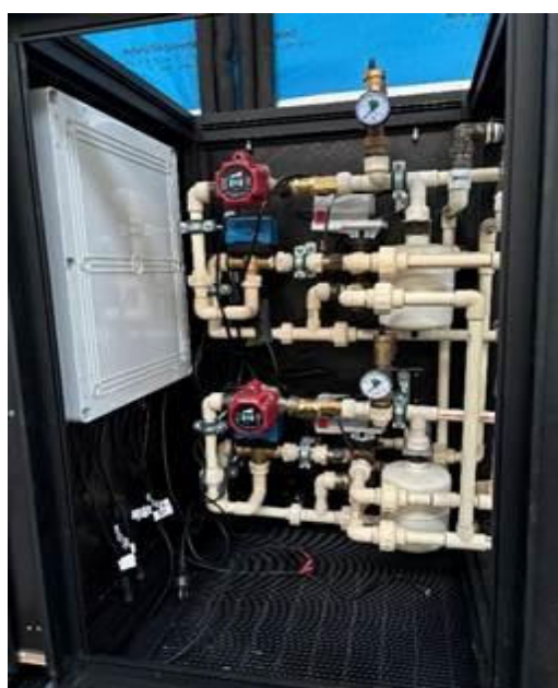
Figure 4. The Hydronic Operations Distribution Module within a Cabinet.
