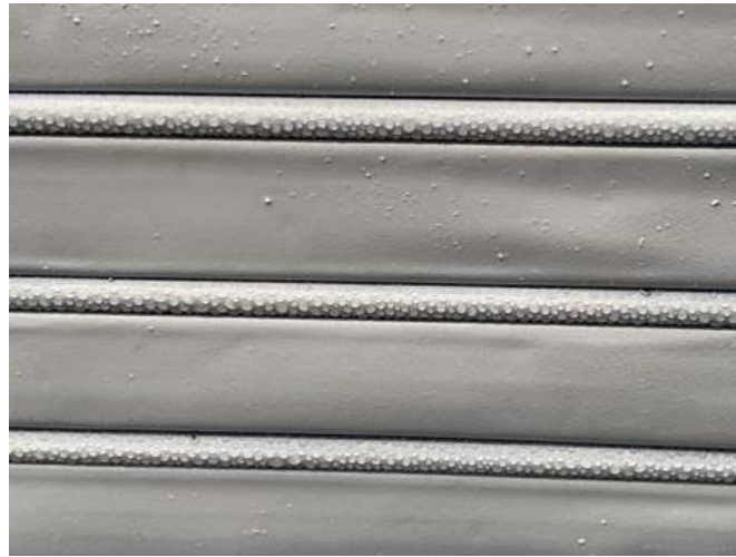
Fig. 14. Condensation on the ‘exposed’ panel of Design 5
